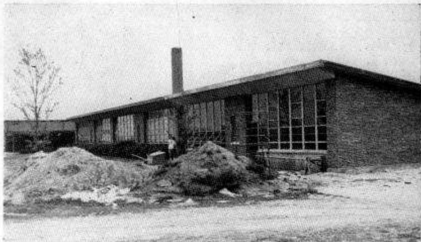
MEDORA ADDITION NEARS COMPLETION — Four Classrooms are being added to Medora elementary school, Valley Station, as part of the overall expansion program designed to relieve crowded conditions which exist in the county system. Six other schools are having additions made this year. All are expected to be ready in the fall.
