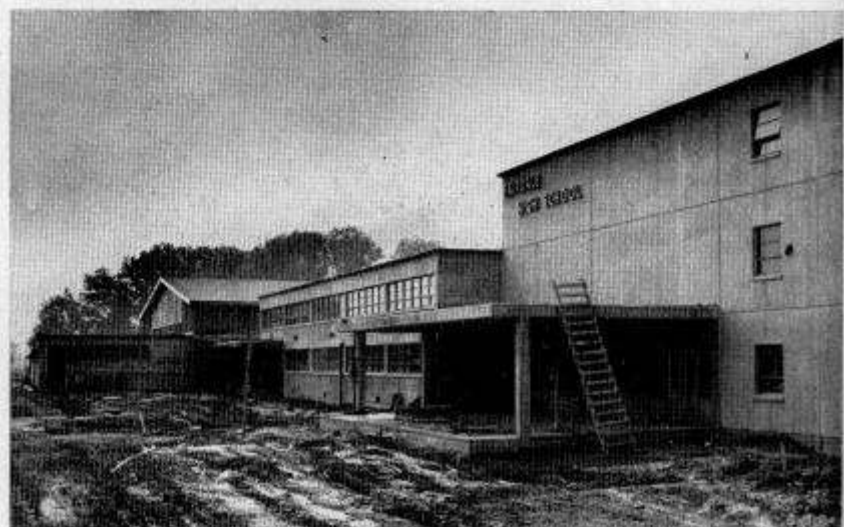
RELIEVES DOUBLE SESSIONS —More than 700 pupils will share this new school home this year. Construction of the Fairdale Junior High School is nearly complete and the facility will be placed in service this month. Use of this building will make it possible for Southern High School to resume regular sessions this year after having scheduled double sessions in 1957-58. The new Fairdale School is located on Fairdale Road. Other new additions to the county school system this year are Pleasure Ridge Park Junior High, Stonestreet Road Elementary School.
